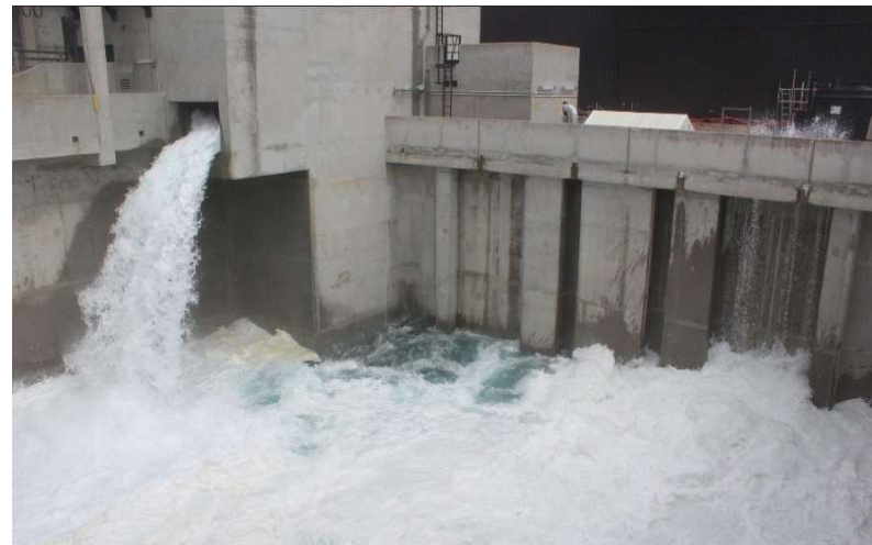
Pump station for trains 1&2 transferred to the operating team
