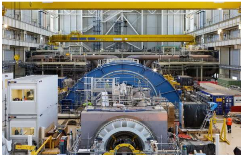
Turbine and alternators in rotation
