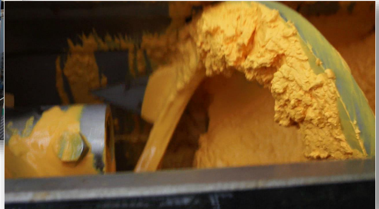
Screw Conveyor, UEC Hobson Processing Plant, Texas
